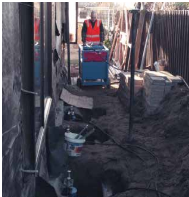
LIMITED TO 1.5 YARDS OF AVAILABLE WORK SPACE, INSTALLATION REQUIRED USE OF PORTABLE EQUIPMENT
